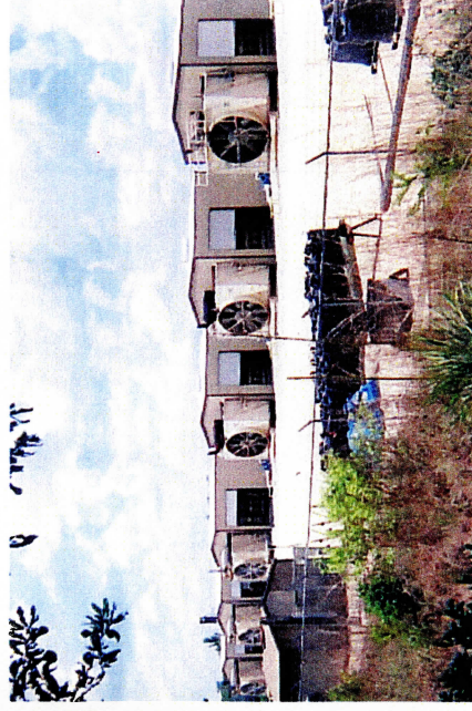
Photo of a gas compressor station.
